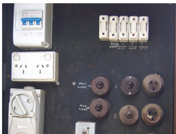
Zelemite backing board to an external switchboard
