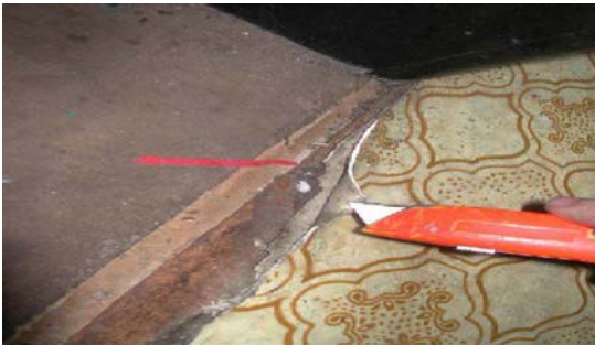
Figure 1 – Asbestos backed vinyl sheet flooring
