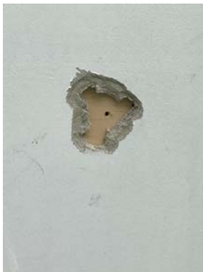
Photo 6: Gap above the patch awaiting filling with a suitable filler.
