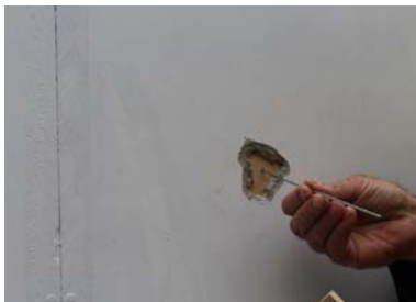
Photo 4: Pulling the sheet against the internal face of the LDB sheet using the wire.
